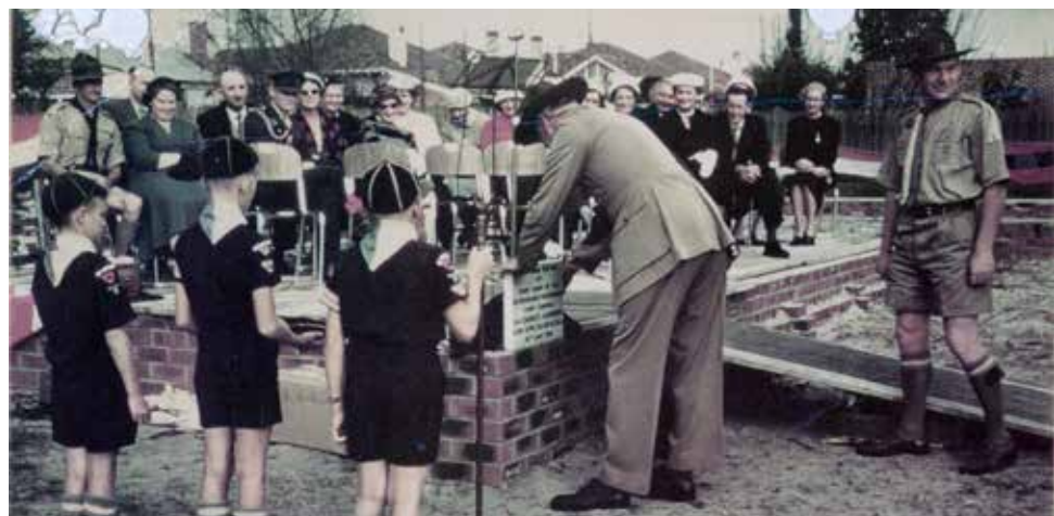
Laying the foundation stone for the Mount Hawthorn Scout Hall, 1958. COV PH05842.
