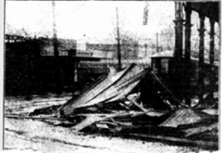
Right on the hill the Rosemount Hotel at North Perth got in the way of the wind last evening and lost its verandah.
