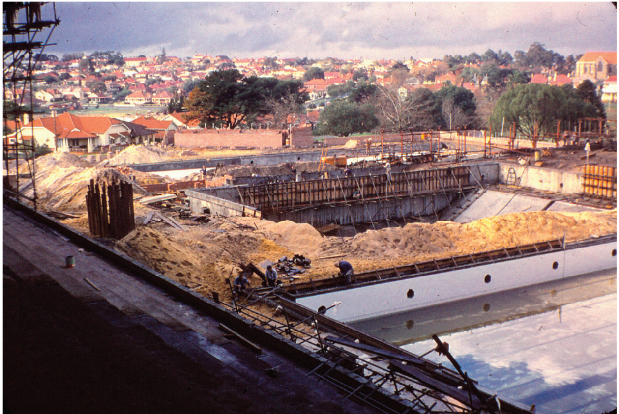
Aquatic centre looking north-east from spectator stands, showing main pool (foreground), diving and water polo pool excavations (centre) and learner's pool (rear), 1962
