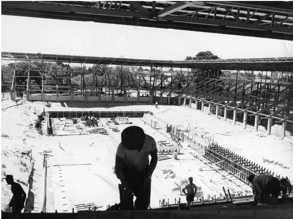
Main pool (55 x 24 yards) and spectator stands under construction, 1962 (COV PH03448 courtesy WASA (Western Australian Swimming Association))
